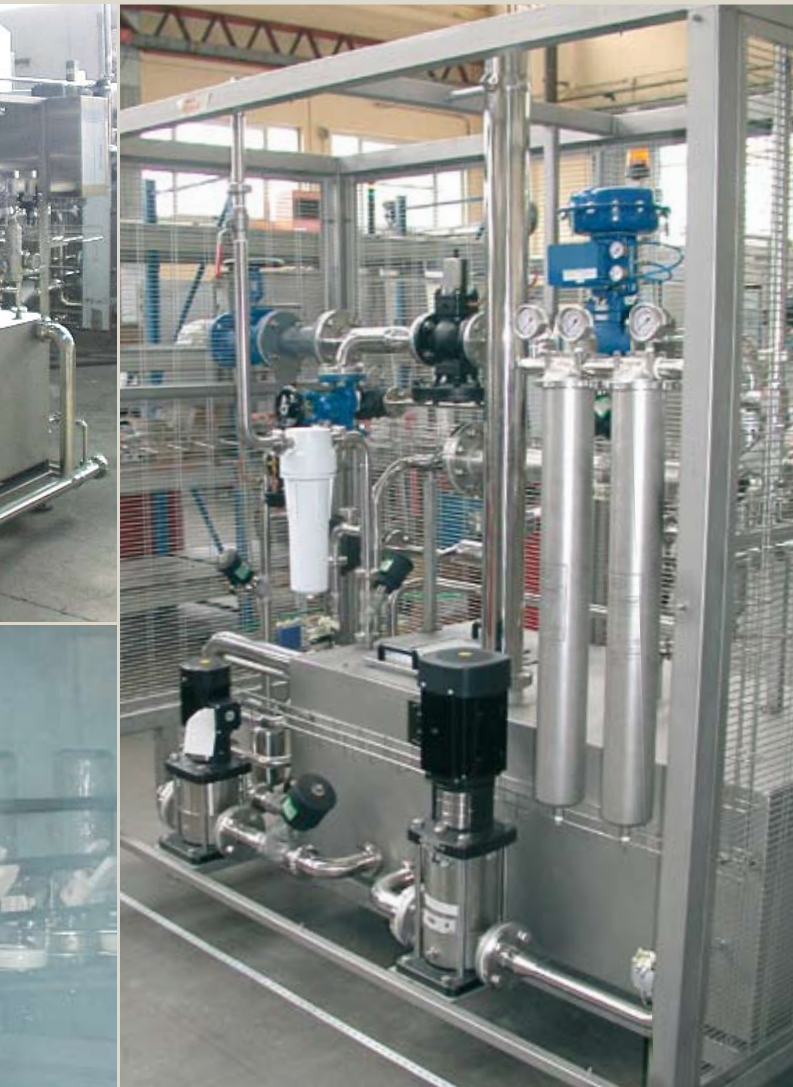
Hot water preparation unit
