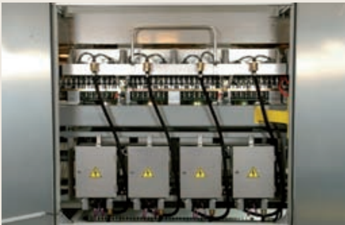
Moving the electric boxes reduces the size of the main electric cabinet.
