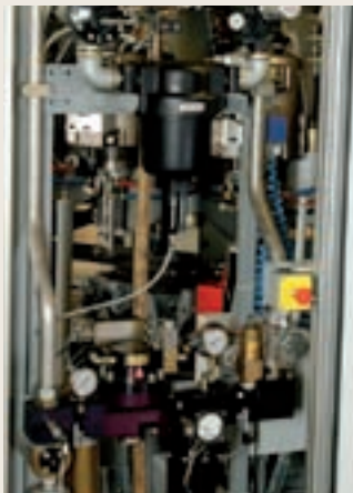
Water and air supply connections are fully accessible.
